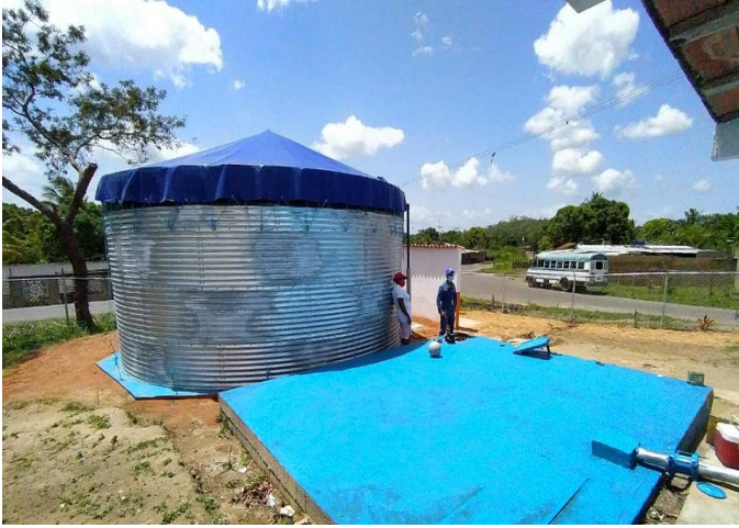
© ALINCA 2021/Saveedra. A 95m 3 water tank installed for the 19 Abril community, located in Bolivar state.
