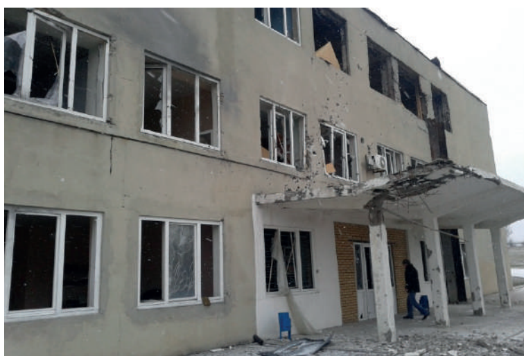
Damaged façade of the administrative office and laboratory building at Donetsk WTP
