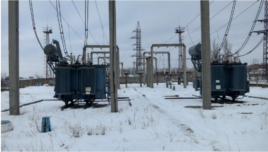
35/6kV main transformer of the outdoor substation of Horlivska WTP 2
