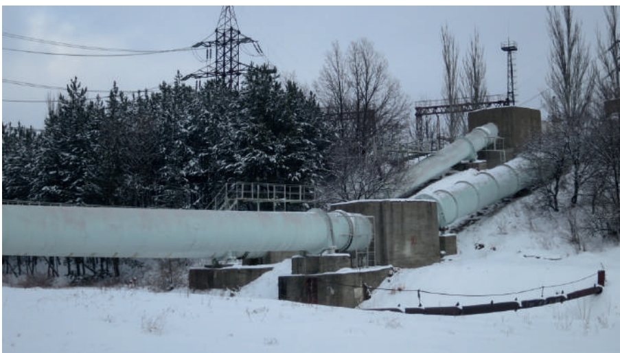
Main pipes after Pumping Station 3A
