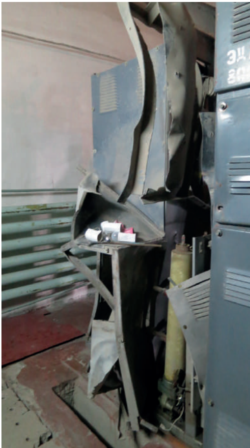
Indoor 6kV Circuit Breaker cell, damaged by shelling
