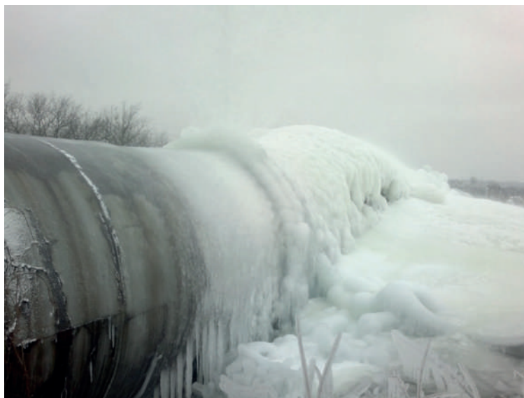
Damaged SDD channel pipeline in winter near Horlivka
