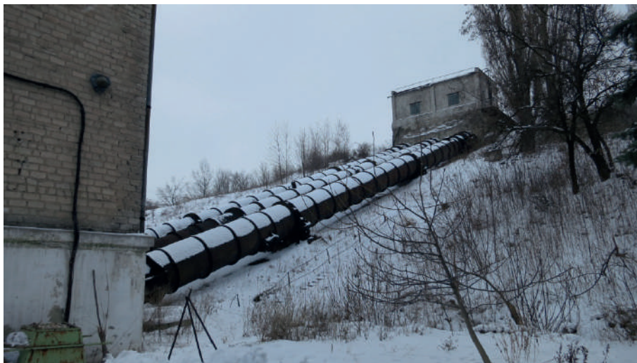
Main pipes after Pumping Station 4
