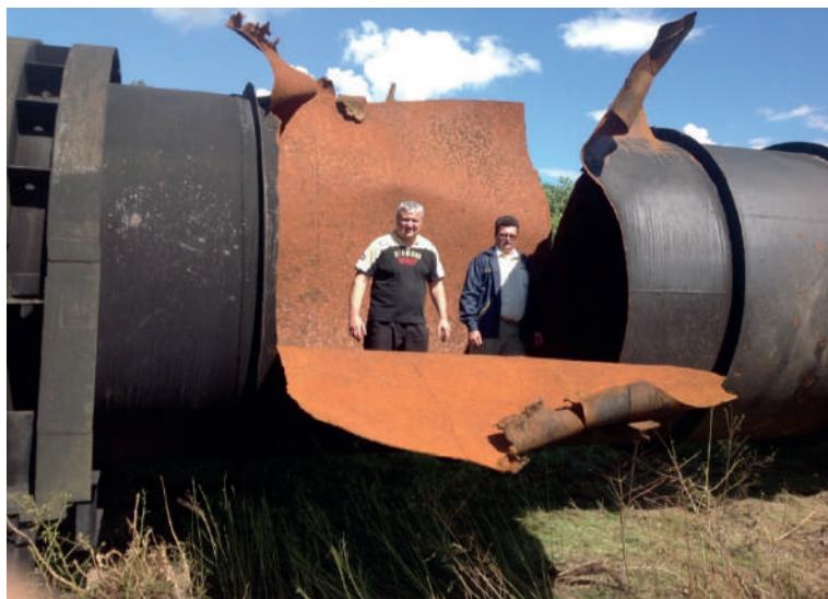
Damaged pressure pipeline of the SDD channel
