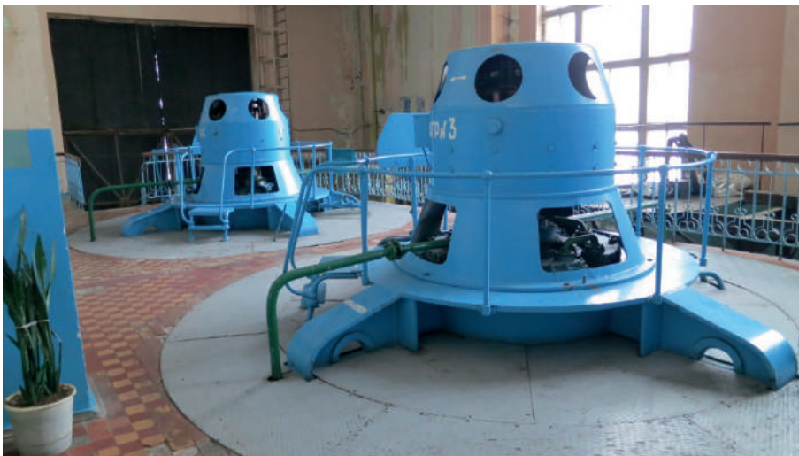
Pumps no. 3+4 at Pumping Station 3
