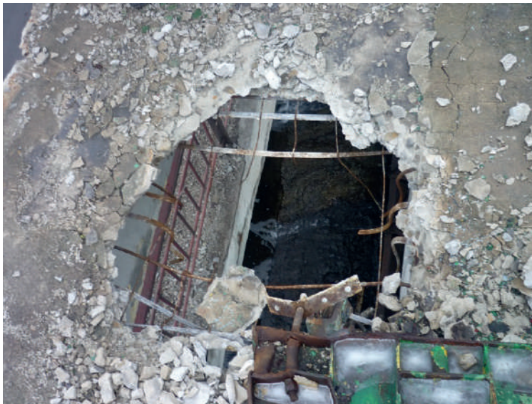
Damages to the Karlivske weir structures of Krasnoarmiyska WTP caused by shelling
