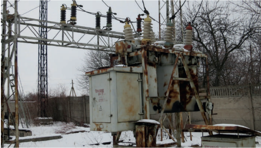
Outdoor 35kV Oil Circuit Breaker, affected by shelling
