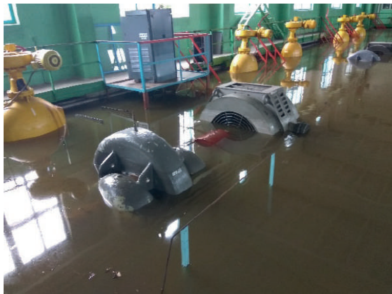
Flooding of 2 nd lift station of the South Donetsk Water Way following unusual operational conditions
