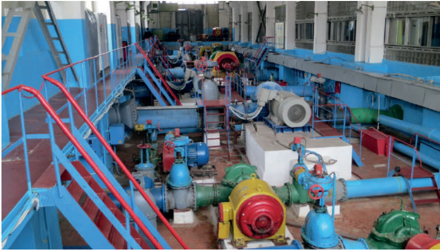
Pumping hall Makiyivska WTP
