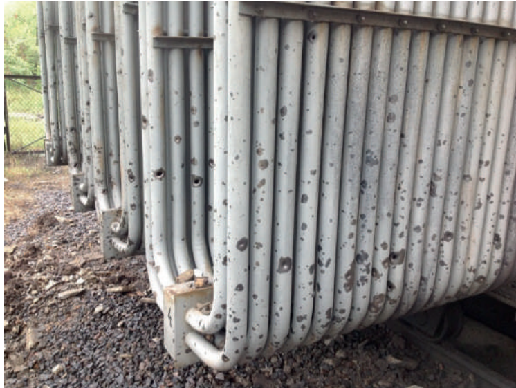
Damages to transformers at 1 st lift pumping station of the SDD channel caused by shelling
