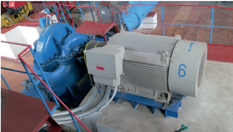
New motor installed in 2013
