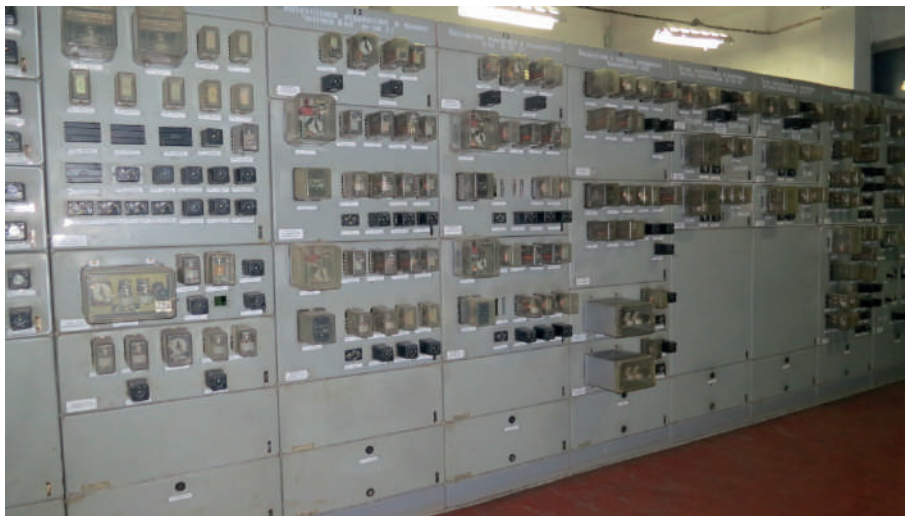
Protection relay board at Sloviansk WTP 2
