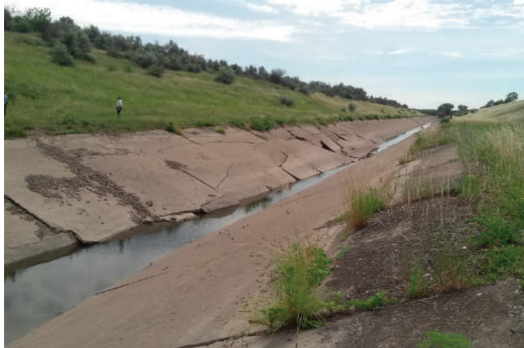
Damages of SDD channel bed following unusual operational stoppages due to conflict
