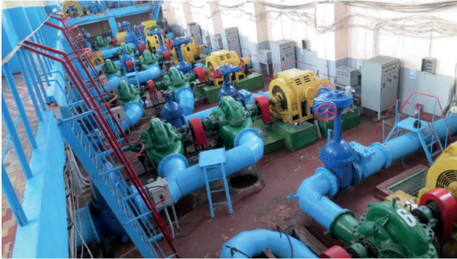
Krasnoarmiyska WTP machine hall
