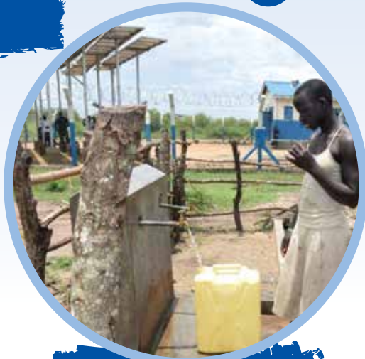
Solar motorised water system
