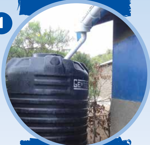
Rain water tank
