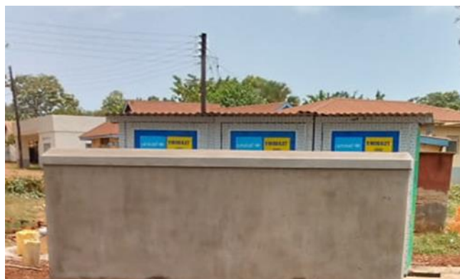
Picture 2: Mobile toilets installed at Jinja Regional Referral Hospital. Picture taken by Paul Kejira
