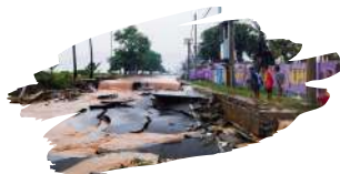
Rádio Renascença/Flood damage after heavy rains, Timor-Leste/ 2021.
