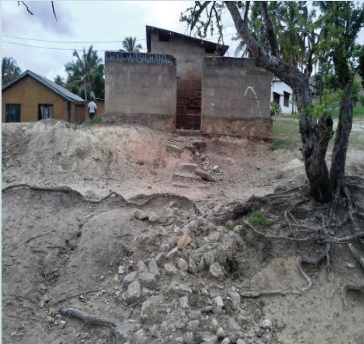
Toilets at an inclusive school in Lindi Municipality. The path to the toilets is too steep with no support for pupils with disabilities.
