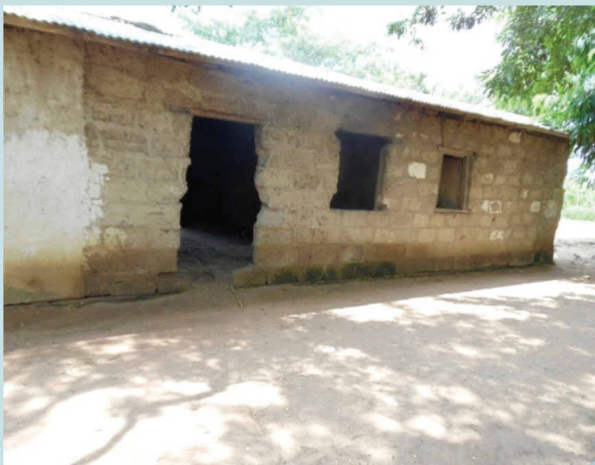
A dilapidated classroom for pre-school pupils in one primary school in Chato District Council. The classroom is also used for cooking.
