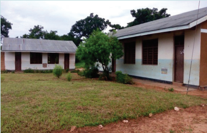
Classrooms built with TASAF funds in one of the secondary schools in Lindi DC
