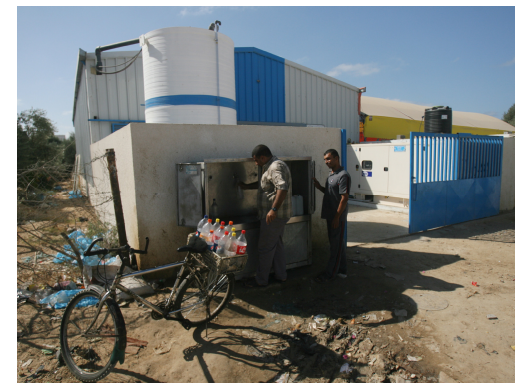
A father fills his bottles with water at the desalination plant built by UNICEF at the Nuseirat refugee camp. UNICEF/EI Baba
