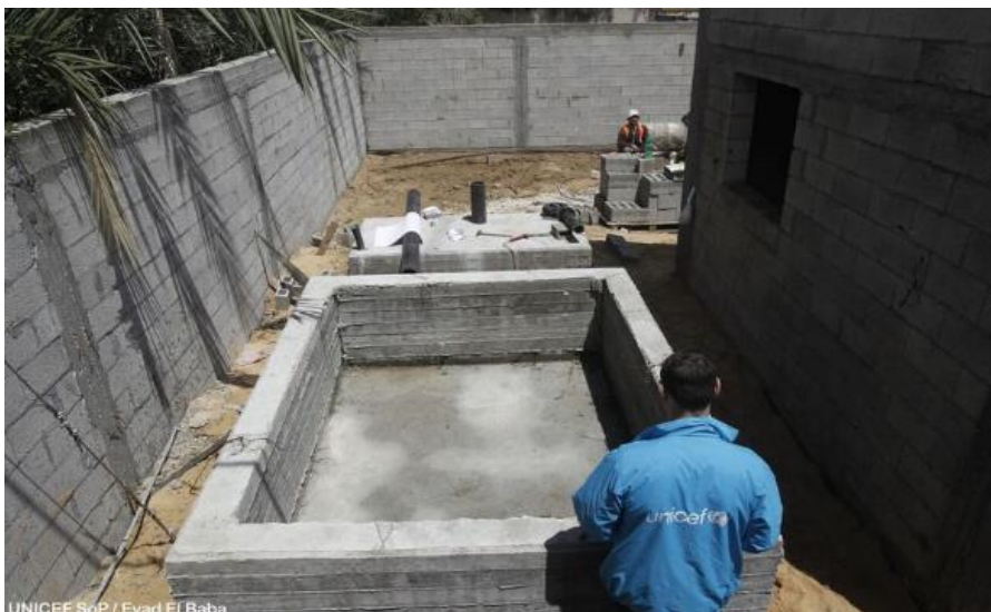
UNICEF field staff visits the water well of Dier AlBalah, in Gaza’s middle area, to supervise the status of construction works.
