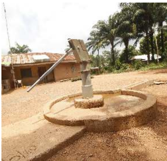
Figure 1: Hand Pump (VLOM)
