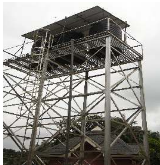
Figure 2: Solar Panels for motorised pumps
