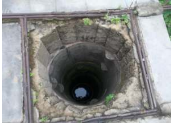
School water well. Credit: Temi 2015
