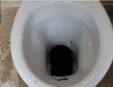
Pit toilet with toilet seat
