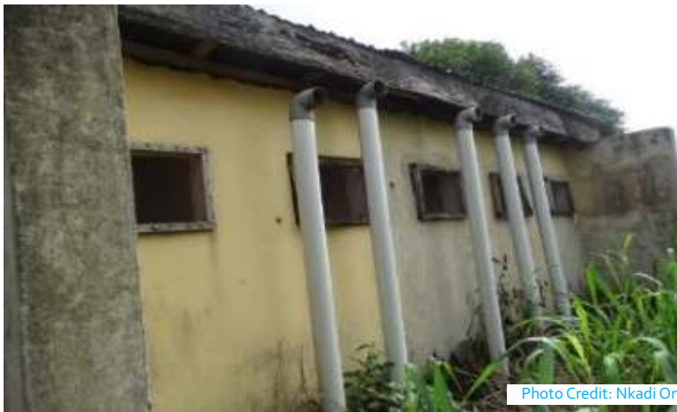
Dilapidated block of toilets
