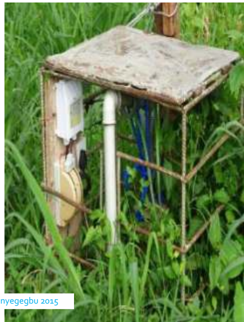
Dysfunctional water borehole
