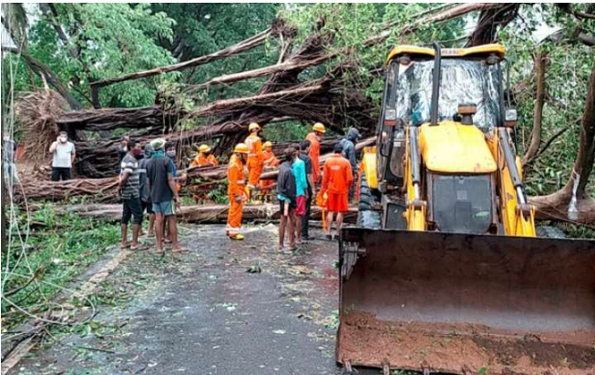
NDRF personnel clearing the fallen trees from road
