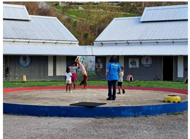
The Providence Infant School in Flankers, St. James, sustained significant structural damage, including the complete destruction of several toilet facilities.
