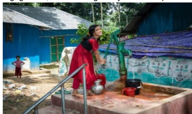
An adolescent girl collects safe drinking water from a climate-resilient raised tubewell in Porshuram, Feni—constructed after the 2024 floods.
