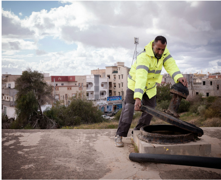
UNICEF/LibyanDesalinationPlant/Zuhair, Tripoli A water technician from General Company of Water and Wastewater (GCWW) operates a desalination plant in Tripoli
