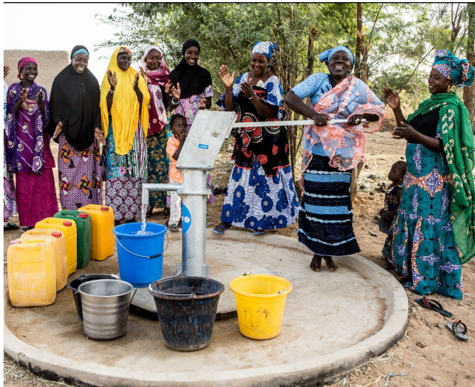
A water pump being built in the village of Dialangou, Mali. Before the construction of the borehole, villagers had no access to clean water within the village.
