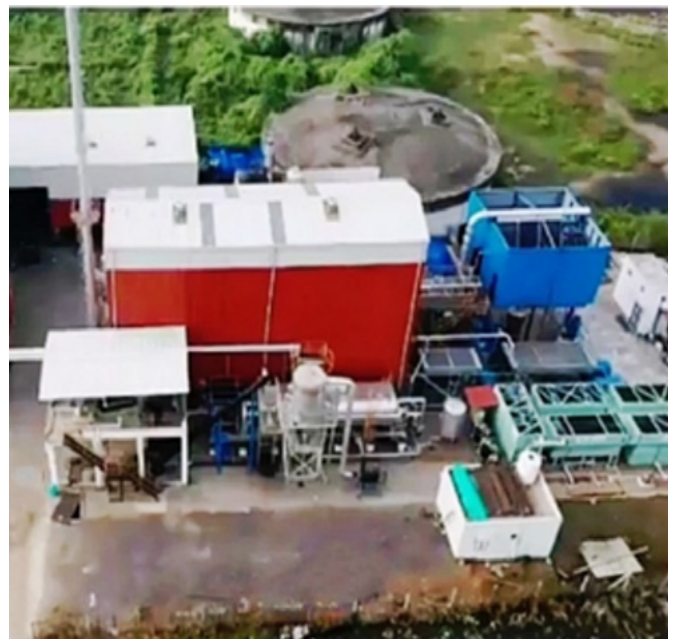
The faecal sludge treatment plant in Vadodara. ©AnkurScientific.
