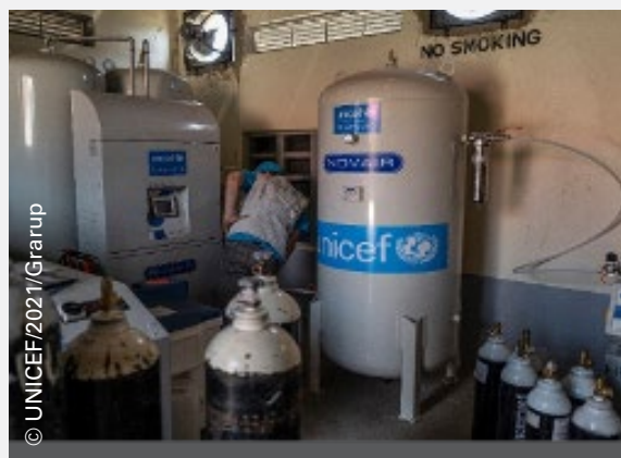
A UNICEF Oxygen Plant-in-a-Box in Soroti Regional Referral Hospital Uganda.
