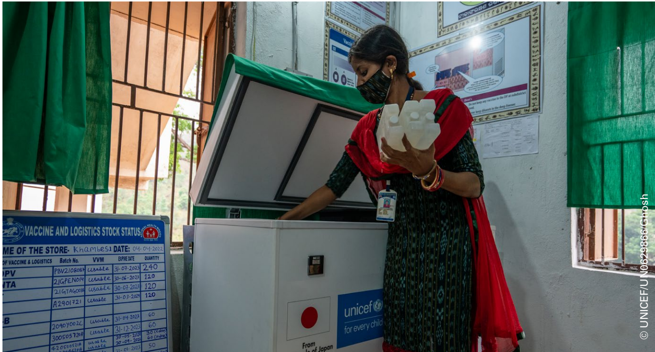
Hiteshwari Behera, ANM and acting cold chain handler, is taking out ice-packs from the deep freezer - a solar direct drive (SDD) vaccine refrigerator, supplied by UNICEF, installed at the Khambesi PHC under Bissam Cuttack CHC at the Rayagada district of Odisha, India. Located almost 83 kilometers away from the Rayagada HQ and about 12 kilometers away from the CHC, the surrounding villages of Khambesi, including the PHC, do not have an uninterrupted power supply.
