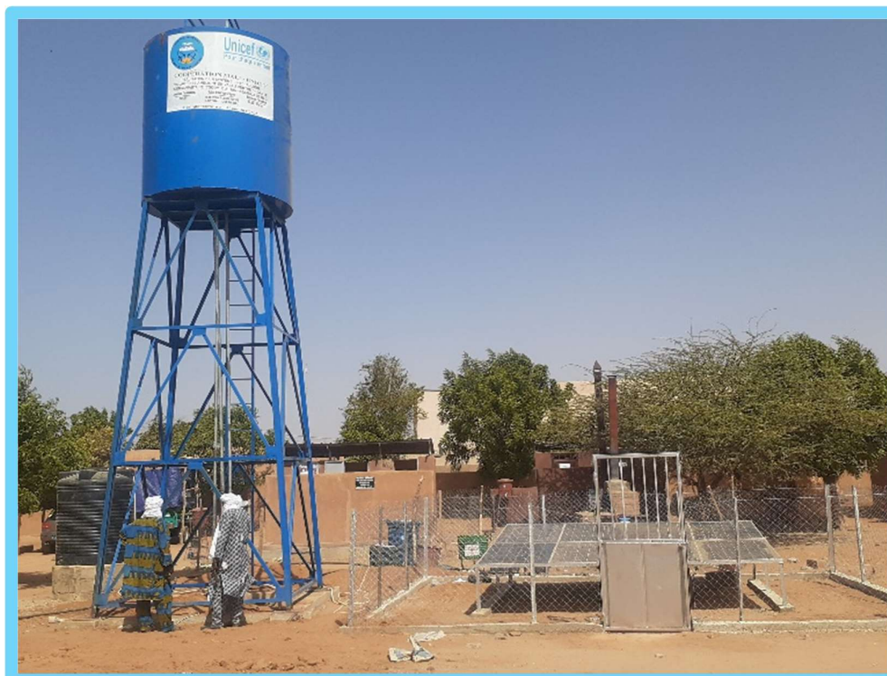
© UNICEF Mali - Water system at the CSCom of Aldjanabandja in Gao region (incl. 1 borehole, 1 water tower of 5 m3, 1 Solar Field of 8 panels; 1 standpipe of 2 taps and a ramp of 4 taps for the population outside the CSCom and 1 washing area, 4 sinks)
