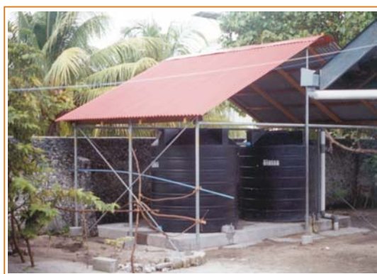
HDP tanks for rain water storage
