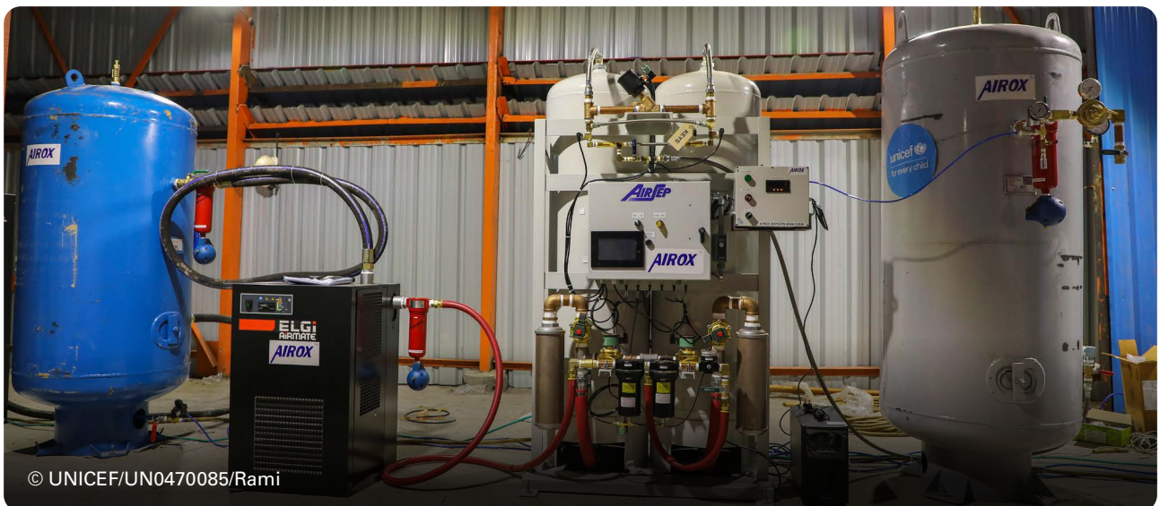
Oxygen Generation plant at Jamnagar, Gujarat.
