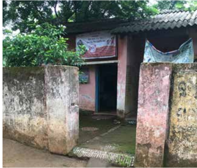
Sub-center with poor infrastructure in a tribal block of Odisha.
