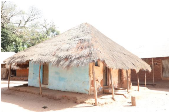
In Guinea-Bissau, traditional homes provide natural cooling due to their design, but are prone to damage and collapse during heavy rainfall and flooding ©UNICEF/GuineaBissau/Mendes/2024
