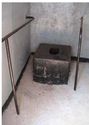
Simple painted metal handrails fixed into the concrete floor and walls. GI / GS pipes and fittings or rolled hollow sections could be used
