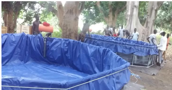
This emergency water plant has been erected to supply water to the COVID-19 isolation and treatment center at Gambella University. It will supply 12,000 liters of water per hour to the center and the surrounding community. UNICEF Ethiopia/2020
