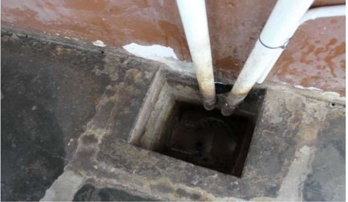
Figure 1: Blocked drainage observed in of the HCFs
