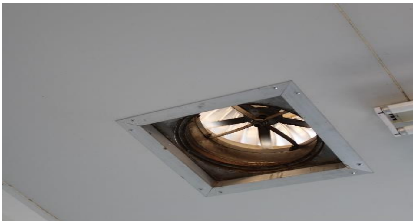
Figure 26: A non-functional extractor observed in one of the HCFs
