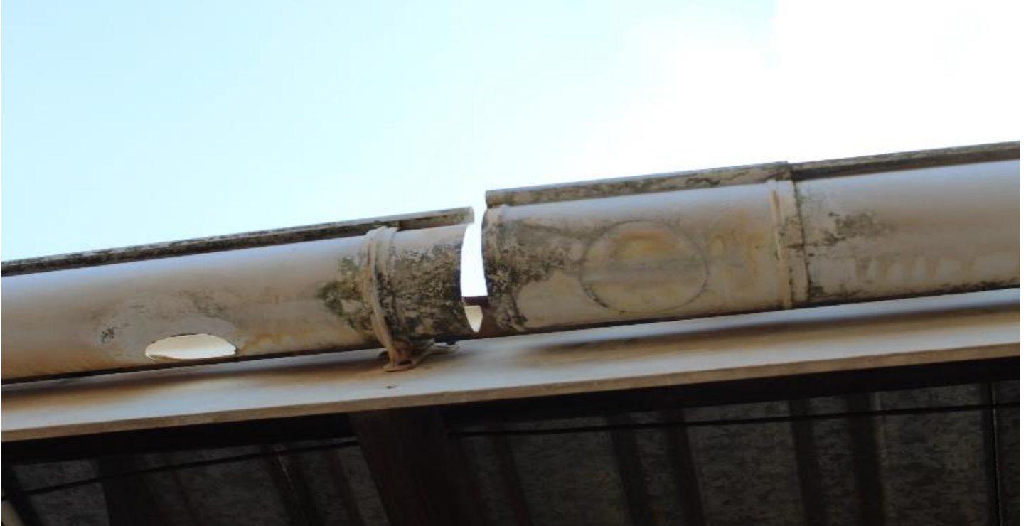
Figure 3 : Damaged gutter in one of the HCFs
