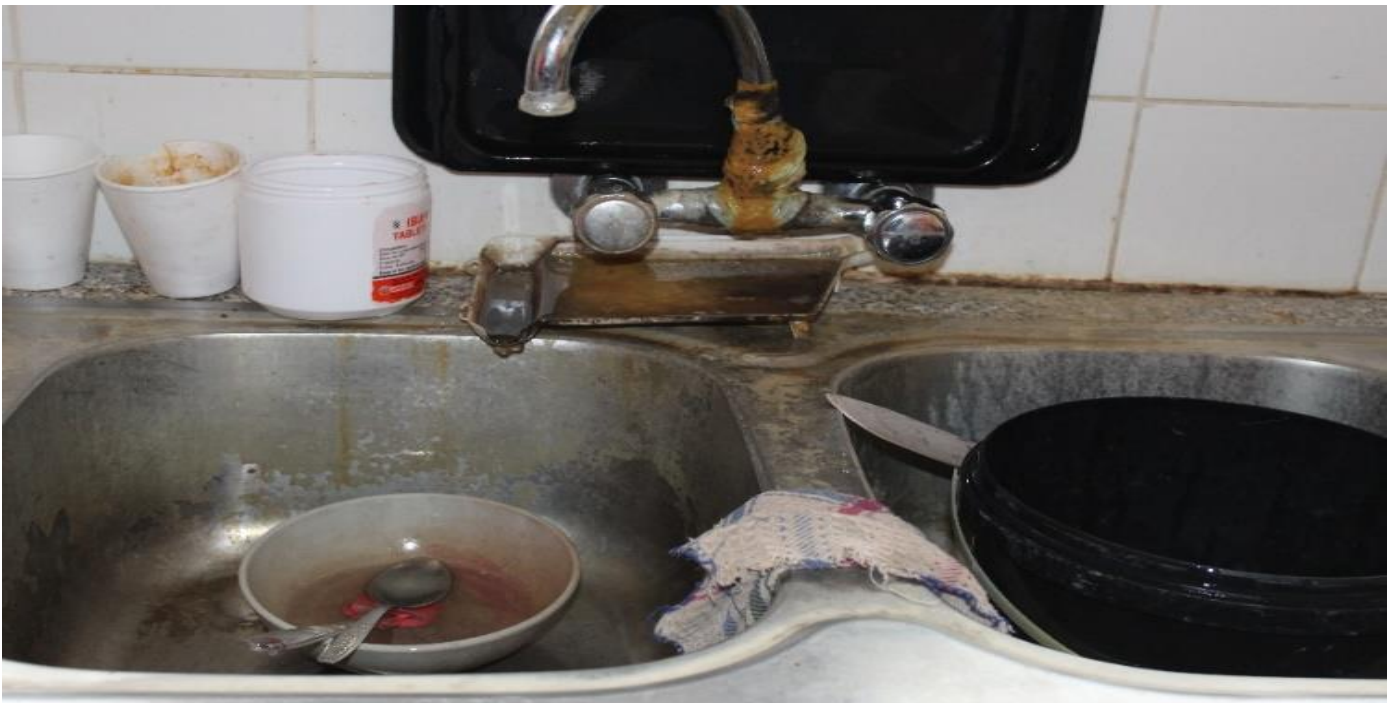
Figure 2: Tap with salt build-up observed in one of the HCFs
