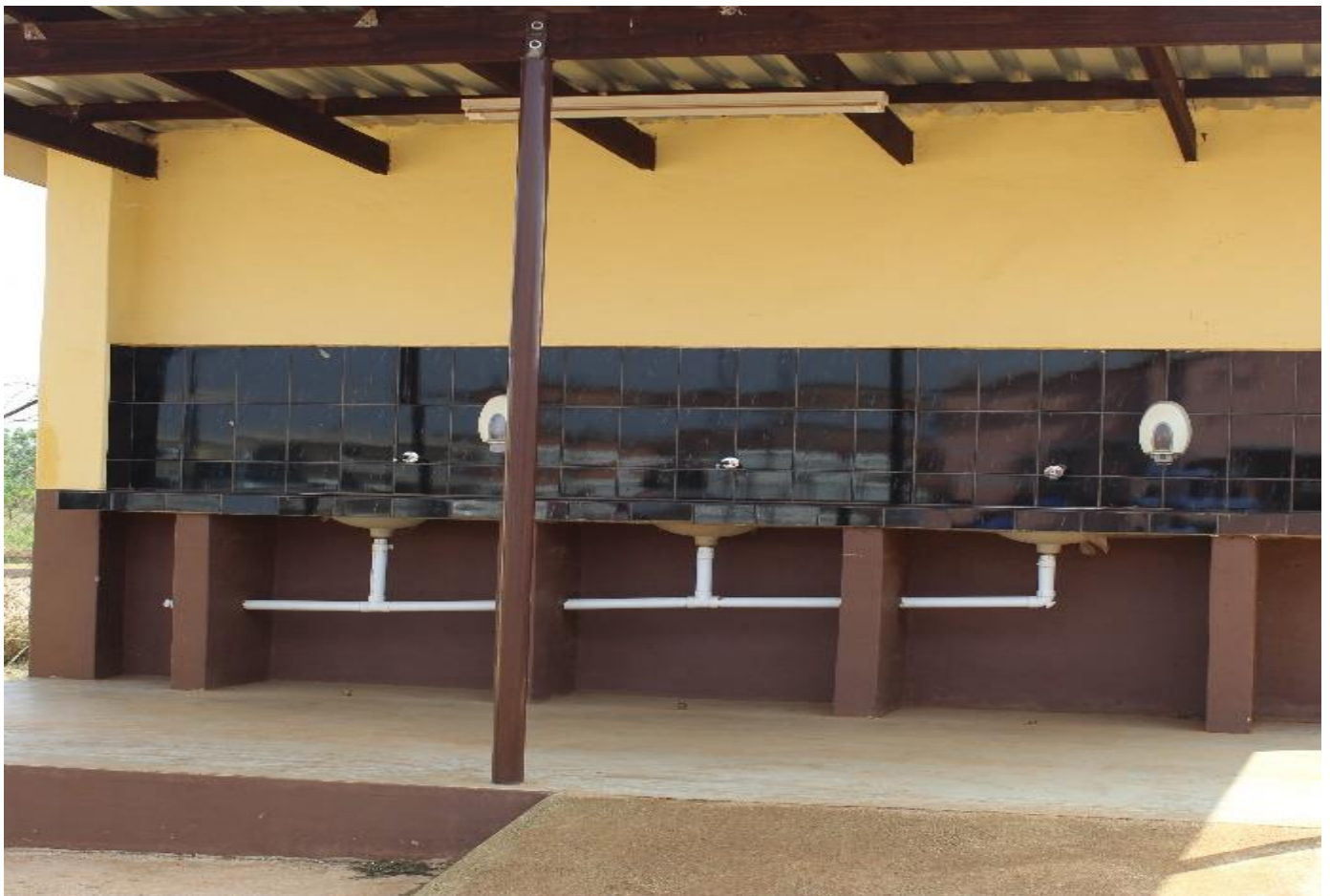
Figure 14: Hand-washing station at one of the HCFs entrance
