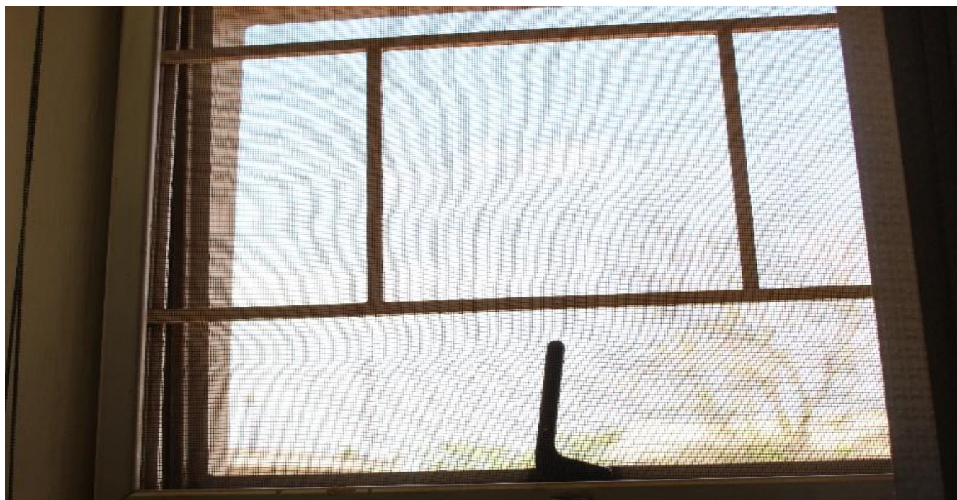
Figure 25: A non-functional window observed in one of the HCFs
