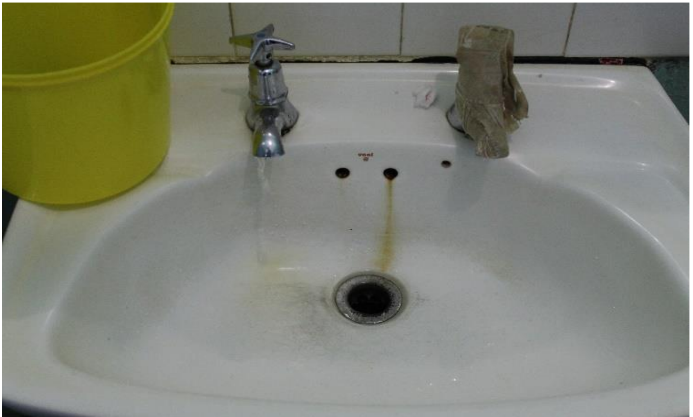
Figure 6: Observed leaking hand-washing sink tap
