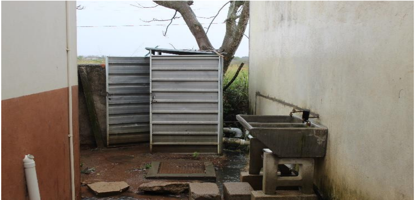
Figure 5: A poorly maintained toilet in one of the HCFs
