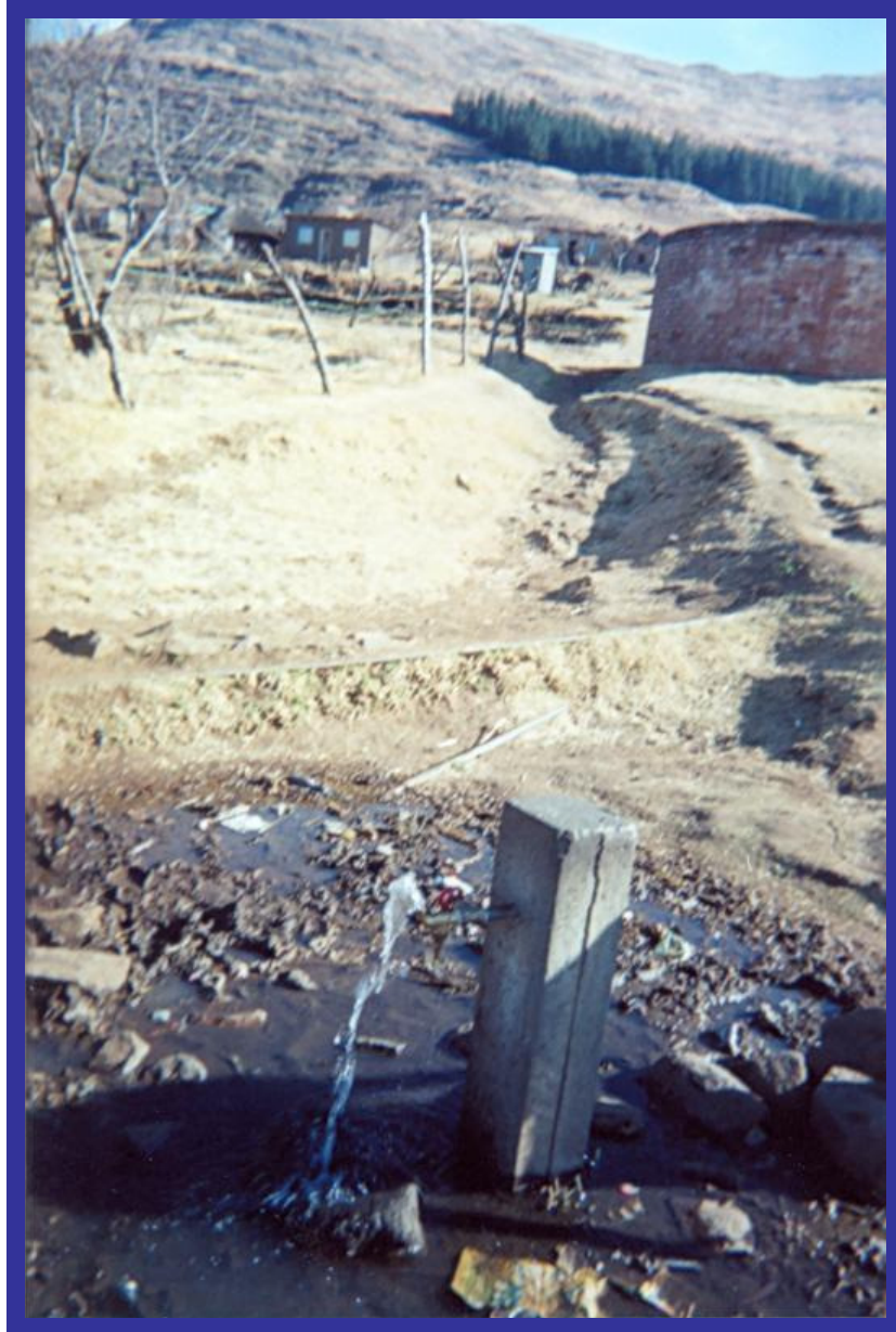
Figure 5.9: Photo of water going to waste
