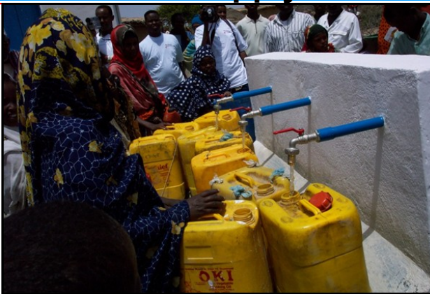
Members of the community in Haraf drawing water from one of the waterpoints supplied through the solar-powered system. © UNICEF/2010/NWZOffice
