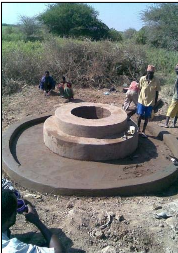
An improved shallow well under construction with EC funding in Middle Shabelle. Credit © UNICEF Somalia/2009
