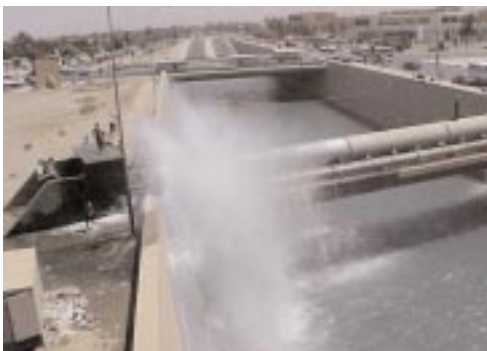
Water gushes out of damaged pipe, filling up the four lane highway underneath.
