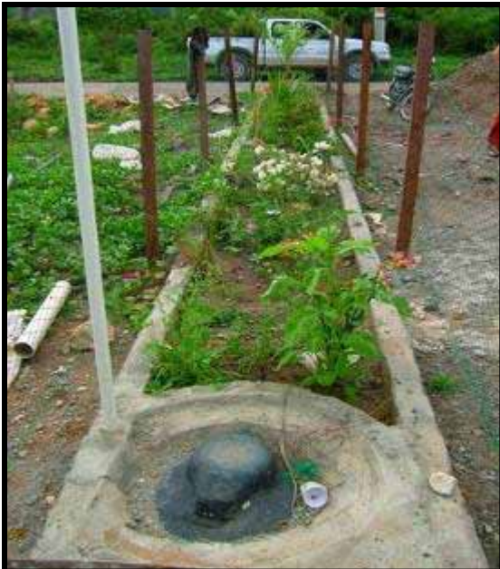
The way it should be: Foreground: top of fiberglass septic tank. Background: vegetated leach field. Result: flowers and vegetables growing from septic tank outflow in narrow land plot.
