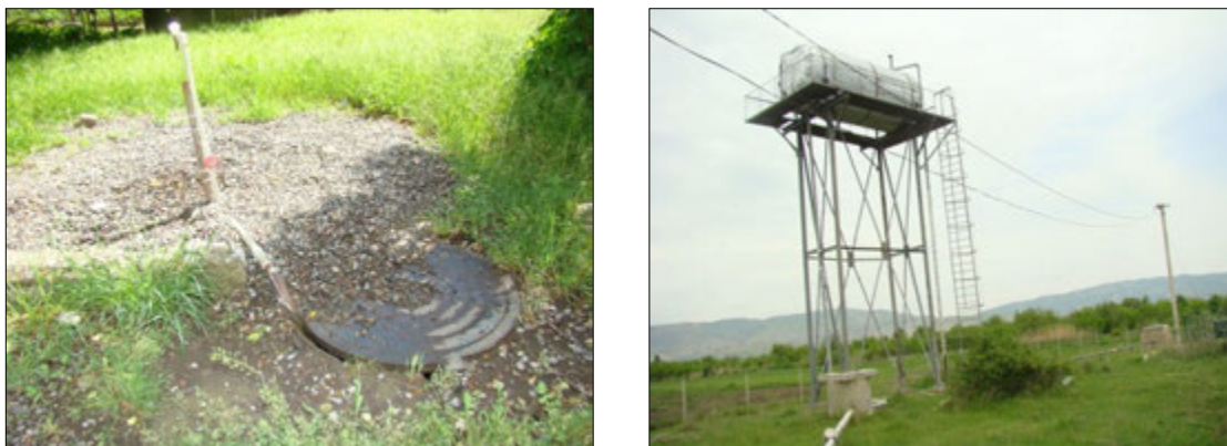
Figure 4 New IDP sites – communal tapstand at a Collective Centre (left) and an overhead tank for supply to a New Settlement (right)
