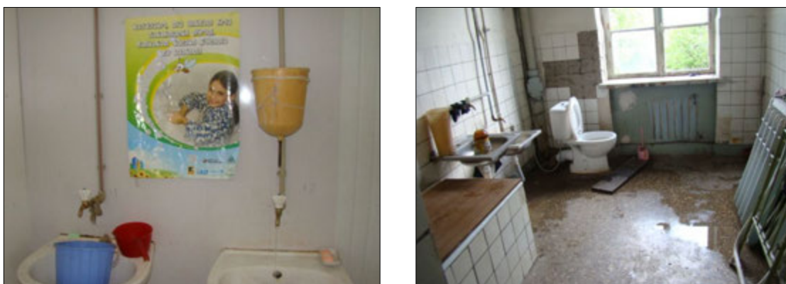
Figure 5 Communal bathhouses in New IDP locations
