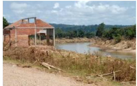
Damaged house beside the Sekong River
