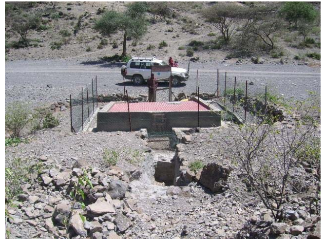
Buried tank for collection of surface water –Photo UNICEF Djibouti-
